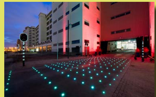
HOV bus lane crossing with RGB LED's in the ground. Strijp-S, Eindhoven. (TCS 6.7)
